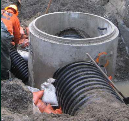
UNDERGROUND SEWERAGE LINE
