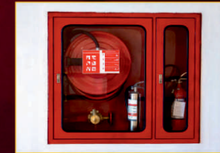
Fire Fighting Systems
