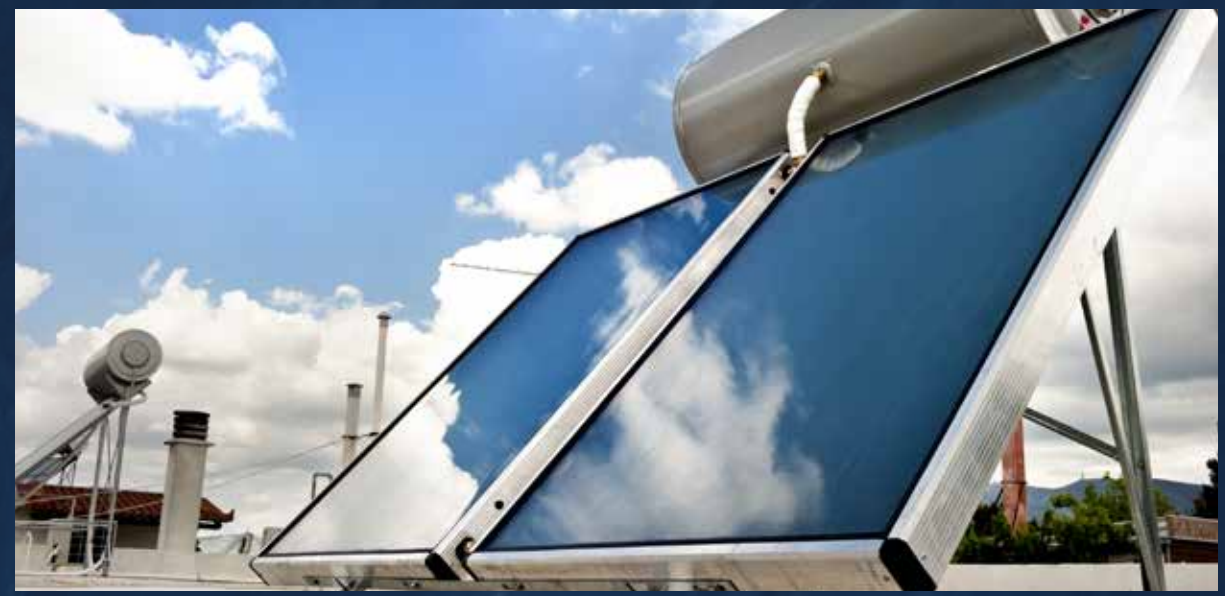
Solar Water Heater
