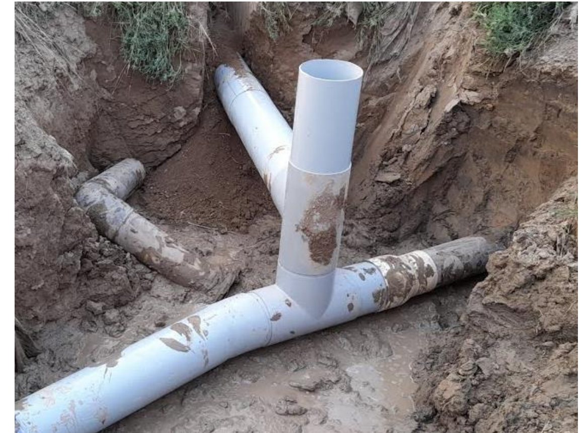
UNDERGROUND WATER PIPE LINE
