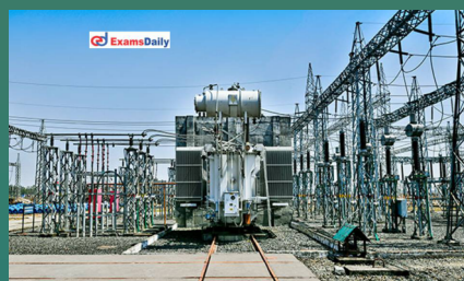
765 / 400 KV Power Grid
