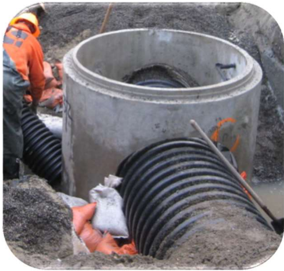
UNDERGROUND SEWERAGE LINE
