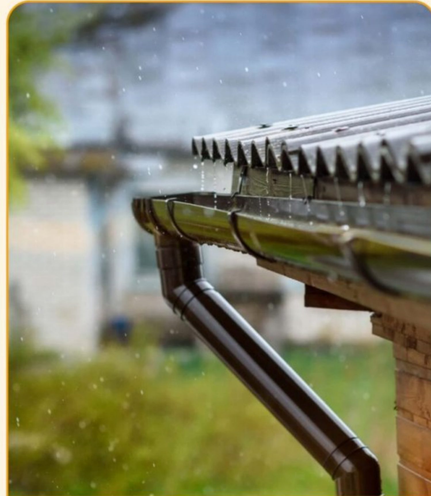
Rain Water Harvesting
