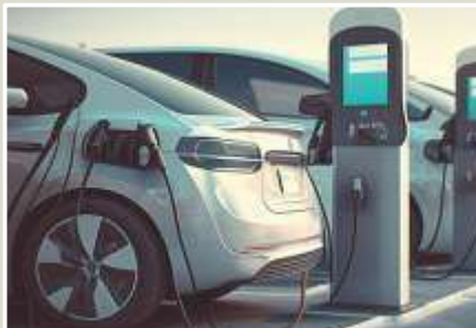
EV Charging Station
