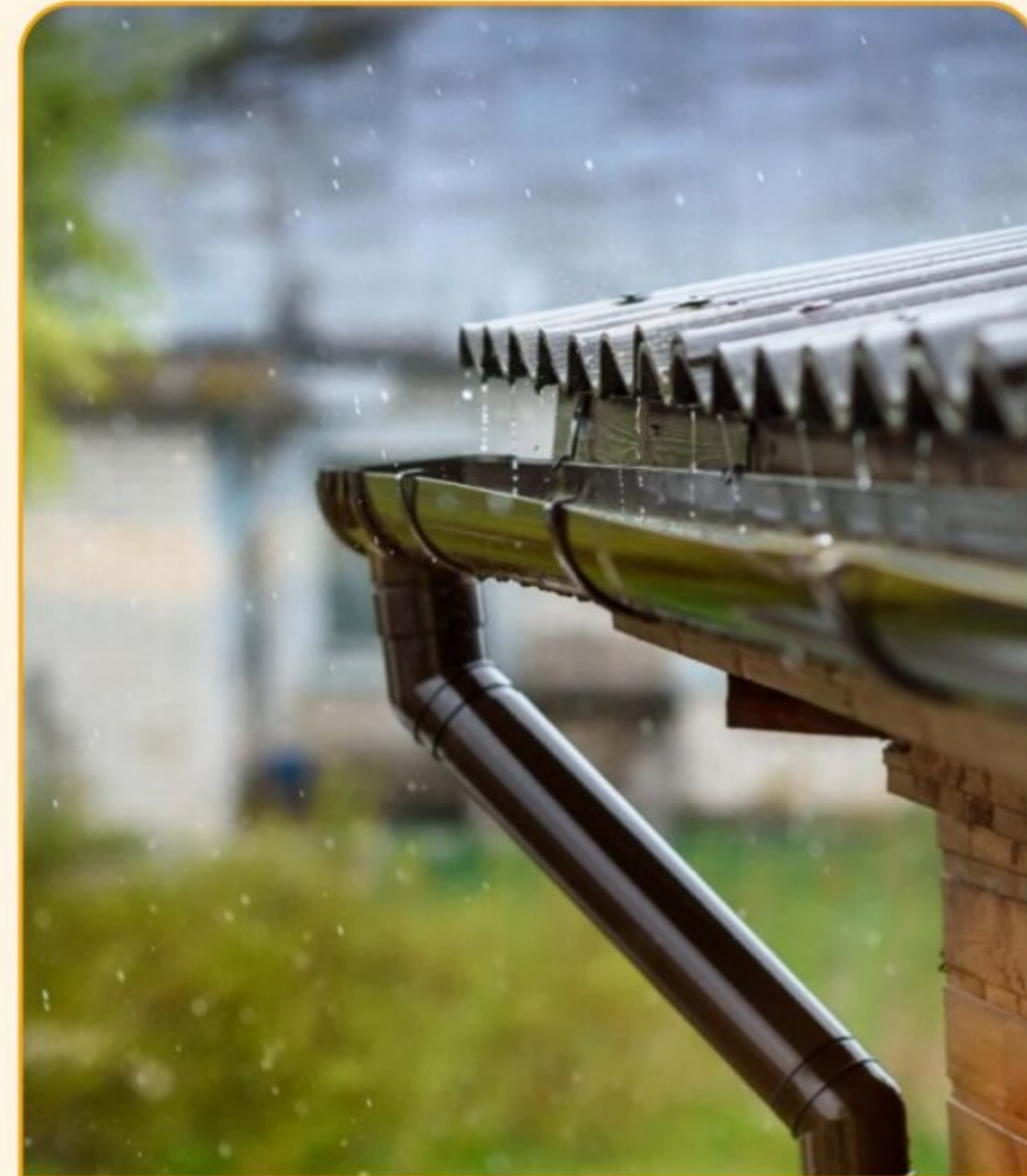
Rain Water Harvesting
