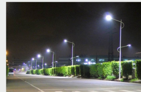
Electrification with Street Light
