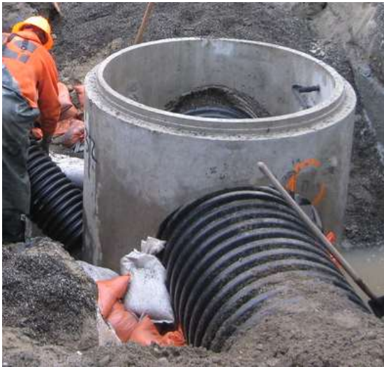
UNDERGROUND SEWERAGE LINE
