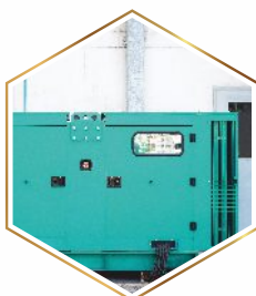
100% power backup in common areas
