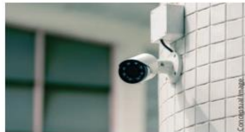
CCTV Camera System
