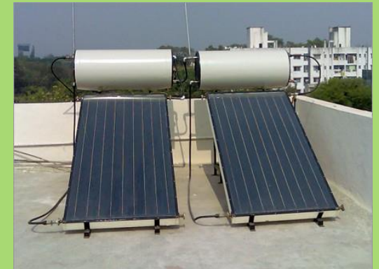
Solar Water Heating
