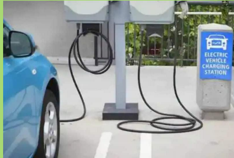
Electric Car Charging Points
