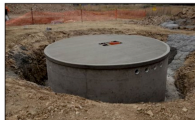
UNDERGROUND WATER TANK
