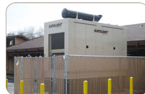
LIFT WITH POWER BACKUP
