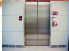
2 lifts with power back-up in each block
