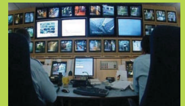
High security CCTV Monitoring
