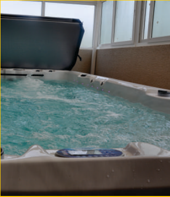
Independent Swimming Pool With Auto recycling unit @ Roof Top
