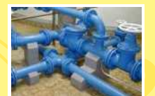
WATER PIPE LINE
